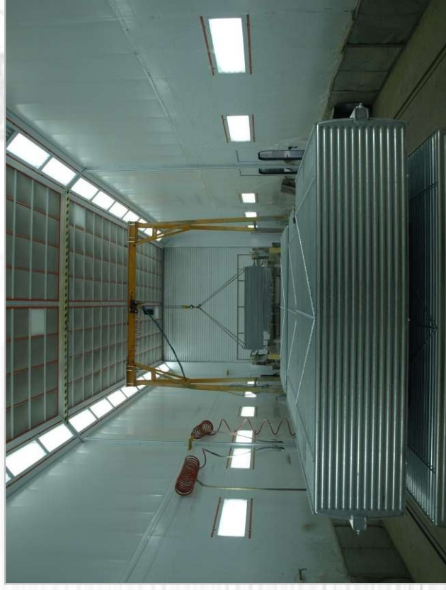
Radiators in paint drying cabin
